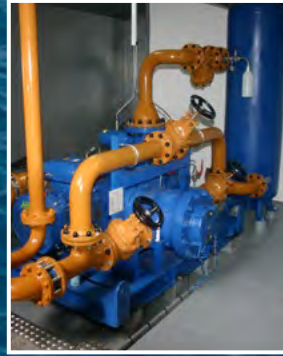
Metering system for diesel measurement
